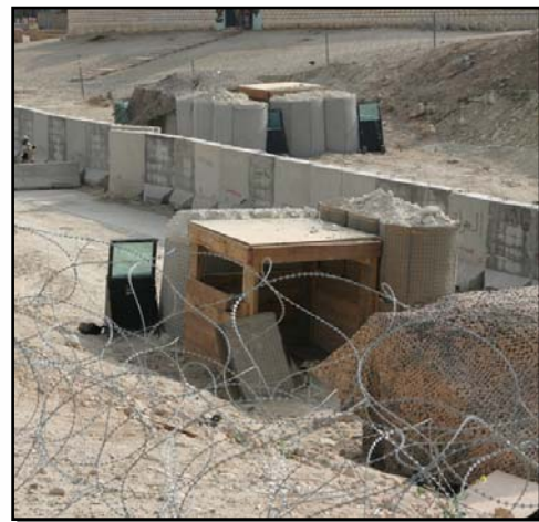
U.S. Marines in Iraq are using Defenshield MDFP's to add visibility and greater protection at fortified entry control and vehicle checkpoints. Photo by Cpl. Zachary Dyer, 2nd Marine Aircraft Wing (FWD)
